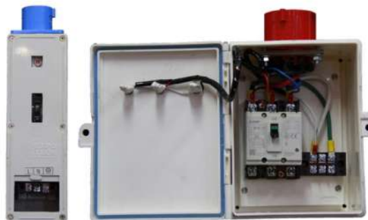
Breaker 15, 30Amp 220V. 50Hz. 1Phase.
